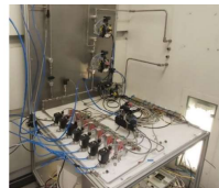
Gas feeding system
